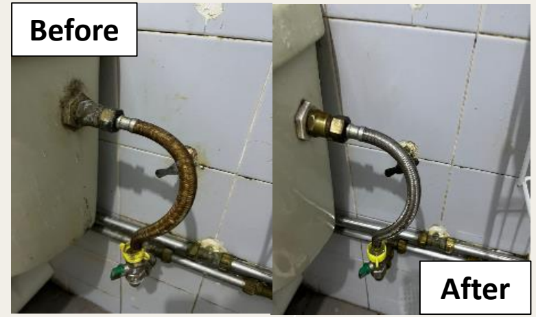
Washroom Stain Surface Cleaning
