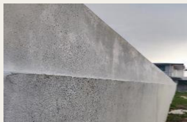
Alkaline Resistant Failure
